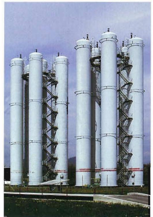
High-pressure cylinders store natural gas in a smaller volume than the low-pressure rigid and telescoping gasholders. The cylinders are in Ljubljana, Slovenia.
