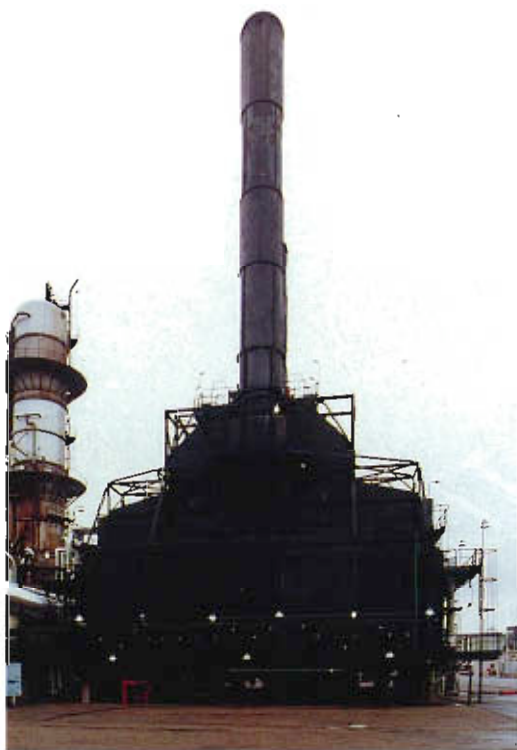
A feed heater at the ChevronTexaco refinery in Pascagoula, Mississippi, heats crude oil to about 700 degrees Fahrenheit. There are gas burners near the bottom of the unit; tubes lining the walls carry the feedstock to the heater. This furnace and another just like it at Pascagoula process 325,000 barrels of oil per day.
