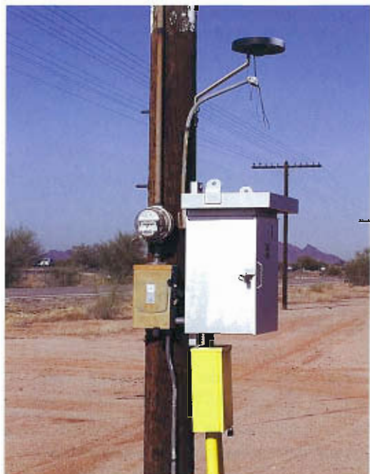
An anticorrosion device along the route of a petroleum pipeline in southern Arizona generates a small voltage opposing natural electric currents that would eat away the metal of the pipe. The circuitry for the protective device is inside the metal box; the black-and-white disk above the box spins when the current is flowing, as an indicator that the system is working.
