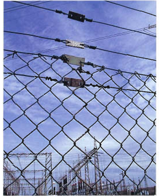
Even the chain-link fence that surrounds a substation has its points of interest. The fence above has a twine thread running through it to block currents induced by power lines crossing overhead. The fencepost below has multiple grounding straps to drain away any stray voltages.
