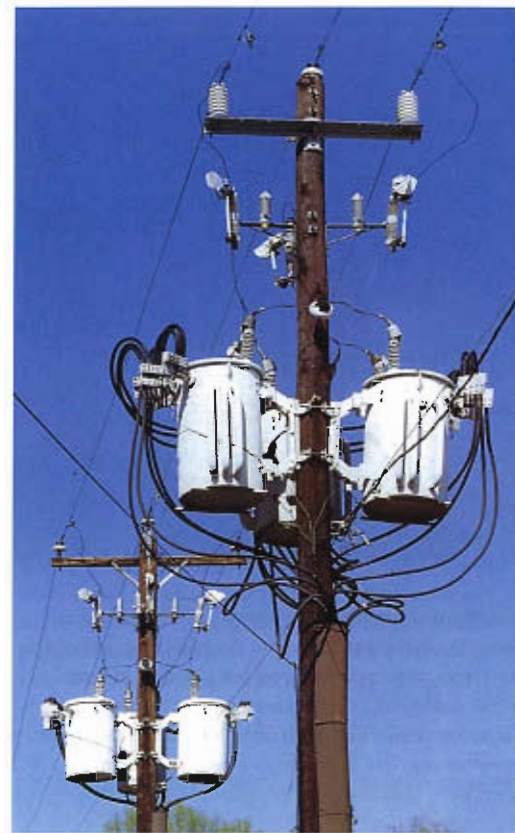
Pole-mounted transformers—also known as “pole pigs”—are such commonplace elements of urban street furniture that we tend not to notice them at all. In residential neighborhoods, there is a transformer for every few houses. The six above supply power to a small shopping district. They are single-phase transformers ganged up in threes to handle three-phase power.
