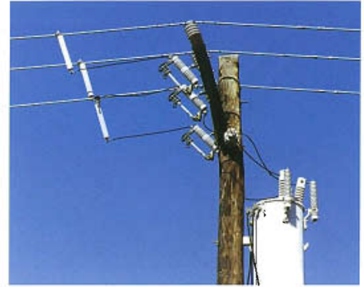
Fuses protect power-line equipment just as they do home appliances. On the pole above, three expulsion-tube fuses are bolted directly to the crossbar; they are wired in series with three silver-sand fuses farther to the left, which serve as a backup. On the pole below, a helpful placard reveals that each phase has two 80-ampere fuses wired in parallel, for a capacity of 160 amps.
