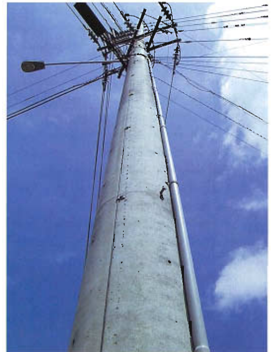
Not all poles are wood: This one, in western Virginia, is made of cast concrete. The thin copper wire running down the surface is a grounding strap.
