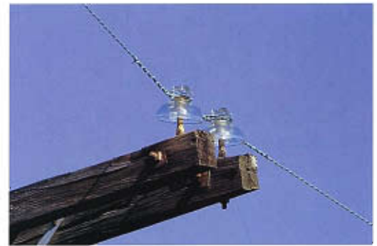
Post-type insulators ( top ) are heavy porcelain castings bolted to the crossbar. Glass pin-type insulators ( bottom ) are now collector's items, but a few are still in service. Here the conductors are also vintage equipment: The green patina shows they are copper, whereas all new power lines are strung with aluminum.
