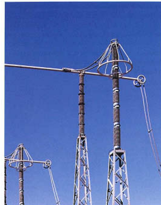
Lightning arresters are installed near every transformer and other items of expensive hardware in a substation. The arrester is the tall strut in the foreground, with the skirt at the top. Ordinarily, the arrester acts as a simple insulator, but when voltage on the system rises to extreme levels, the arrester becomes a conductor, shunting the excess current into the earth. The strange lampshade at the top is an arc ring, meant to limit the damage if a lightning bolt “flashes over” from the arrester to the ground.
