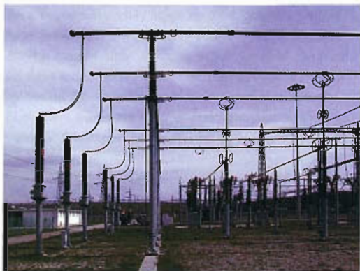
A substation “bus” is a set of parallel conductors that carry electric current from one component to the next. Here two buses (with a total of six conductors) are formed out of aluminum tubing held aloft on insulated pedestals. The columnar devices at the left are instrument transformers that monitor voltage on the two buses. The substation is in Redipuglia, Italy.
