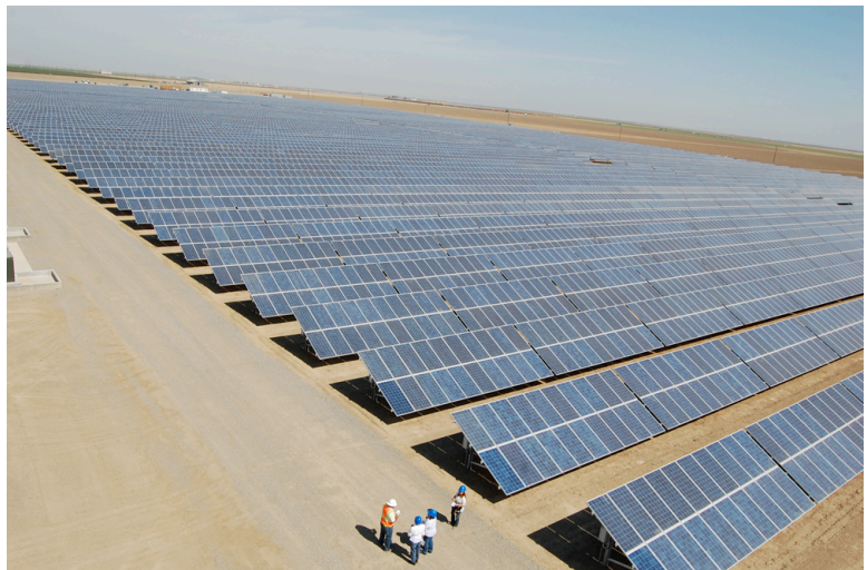
18 MW tracking solar PV installation at Five Points, CA. Image: Blue Oak Energy
