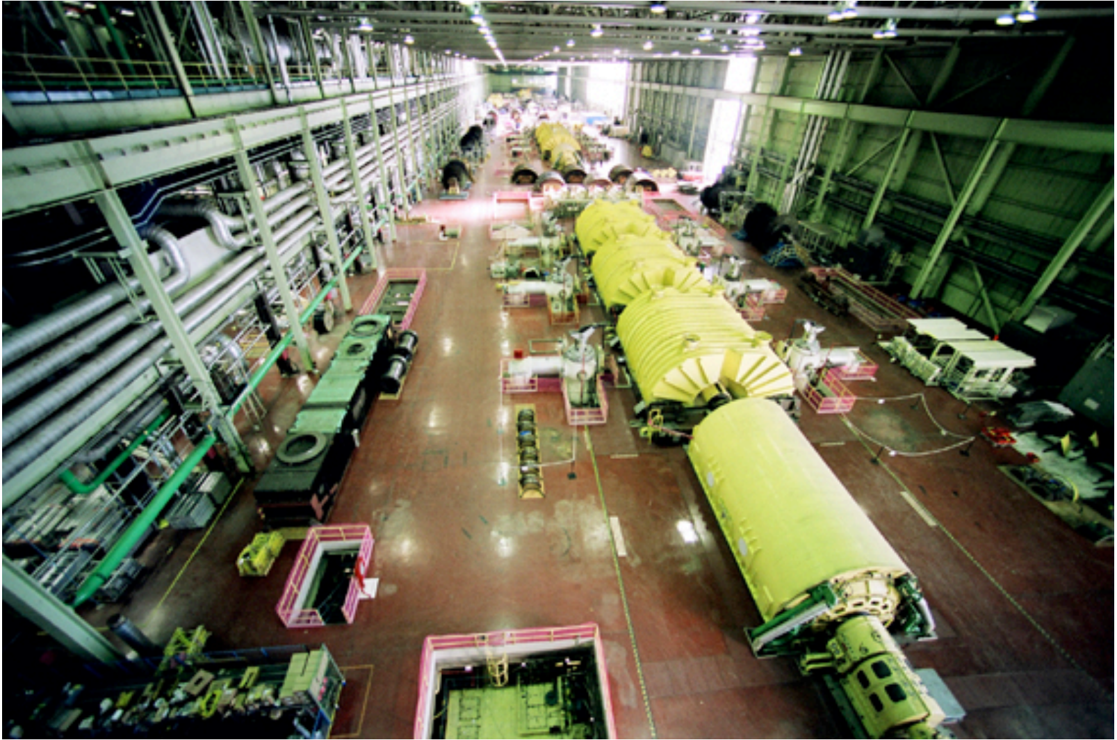
The turbine hall of Bruce Power's Bruce A nuclear power plant in Ontario, Canada.
