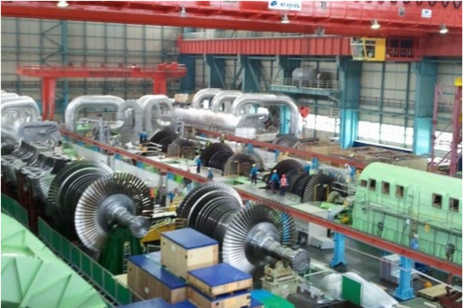
Alstom steam turbines, Ulchin Nuclear Power Plant, S. Korea ( copyright unknown )
