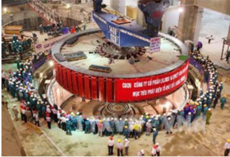
15 m rotor for 400 MW generator at Son La hydroelectric facility, Vietnam (L). Rewinding the rotor for a small hydroelectric plant (R)
