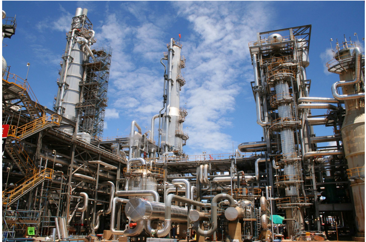
Fertilizer plant ammonia and urea production
