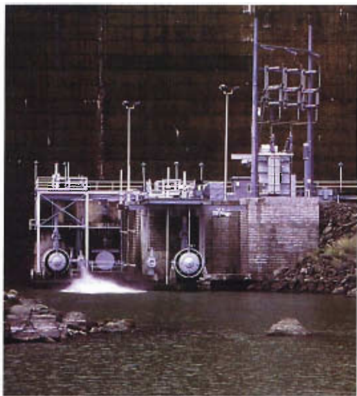
A small hydroelectric installation at the base of the Monticello Dam west of Sacramento, California, exploits a high head (about 400 feet) to extract about 11 megawatts of energy from a modest flow of water. The turbine is a Francis wheel, a hybrid type that draws on both the impulse and the reaction principles. The discharge is above the level of water in the tailrace.
