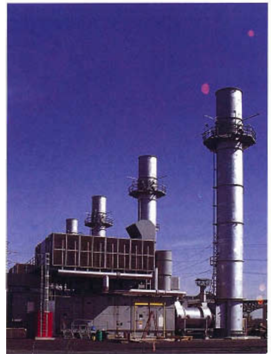
Four new combustion turbines in Kearney, New Jersey, are seen under construction in 2002. The air intakes are atop the buildings that house the turbines.
